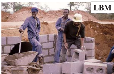
Blockwork has been used successfully for simplified construction of headwalls on small culverts and for the support of concrete slabs to make a box culvert.
