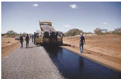
Visual control of the bitumen distributor and continuous inspection of the work on site are important parts of the quality control procedures and can reduce flaws in thin seal that could lead to premature failure of the surfacing.
