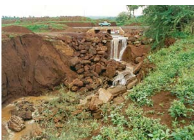
Erosion in outlet channels can cause considerable environmental damage in sensitive areas.
