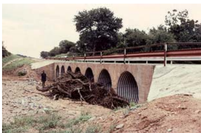
Banks of pipe profiles culverts are prone to blockage by trees even when large sizes are used.
