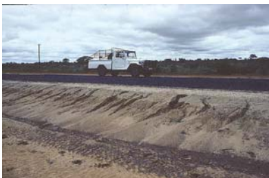
Severe erosion of side slopes that can lead to siltation of streams and rivers.
