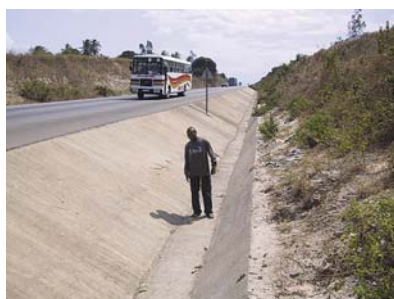
Deep V-type drainage ditches leave no room for recovery if a vehicle runs off the road.
