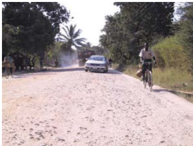
Due to loss of fines, gravel roads often become very rough which make driving conditions hazardous and, in addition to severe driver discomfort, impose very high vehicle operating costs.
