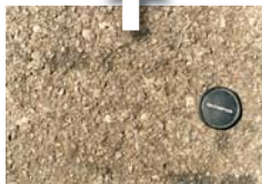
Loss of second seal due to bitumen hardening and embrittlement.
