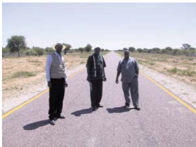
An example of a single Otta seal with a sand seal performing very satisfactorily after more than 13 years in service and without any surfacing maintenance in a harsh environment.
