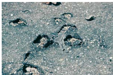
Salt damage may appear in the form of “blistering”, “doming”, “heaving” and “fluffing” of the prime or surfacing.
