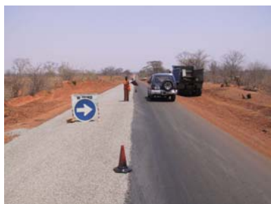
Resealing is a typical periodic maintenance activity.
