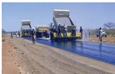
A typical surface treatment operation - spraying a thin layer of bitumen onto a road surface prior to the application of aggregate.
