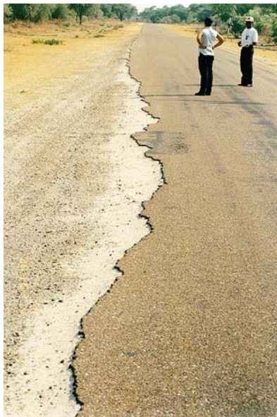
Severe edge break on a 5.0 m carriageway even at relatively low traffic levels (< 100 vpd).
