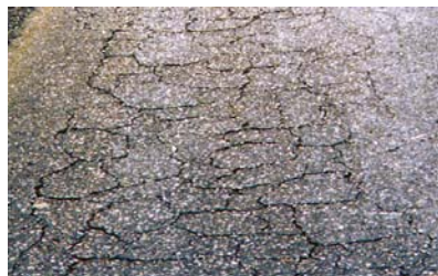
Cracking of surfacing mainly due to oxidation and consequent hardening of bituminous binder.
