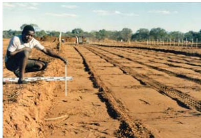
Collapse settlement in excess of 150 mm after impact rolling.
