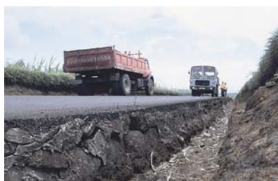
Road safety audits help to produce designs that reduce risks to road users.
