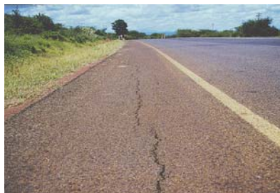
Typical longitudinal cracking caused by large volumetric changes in an expansive soil subgrade.
