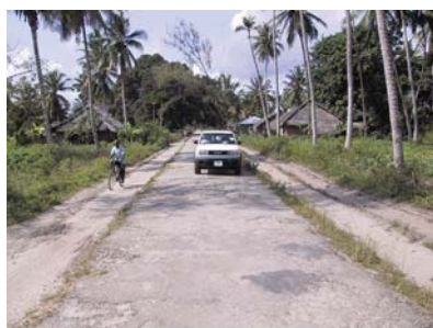
A road where one or more of the seven dimensions of sustainability is missing.
