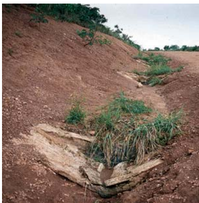
Concrete scour checks in side drain.
