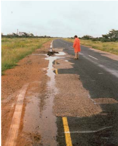
Water infiltration in shoulder and rut leading to edge failures.
