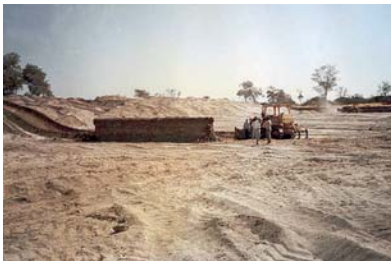
Large thickness of overburden does sometimes exclude labour-based methods for winning gravel materials. (The example shown in the picture is from construction of LVSRs where the thickness of the overburden is in excess of 2 m).
