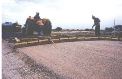
Drag brooming is sometimes applied in order to improve distribution of aggregate.
