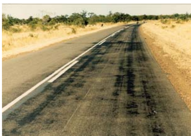
Bleeding due to embedment of surfacing aggregate in base.
