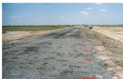
An example of severe distress to a runway surfacing due to salt attack resulting in damage within two years of its construction.
