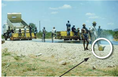
Having spray cans with bitumen emulsion available at all times during surfacing operations for repairing minor faults is part of good quality assurance.
