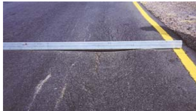
An example of rutting due to permanent deformation of the base layer caused by densification of material.
