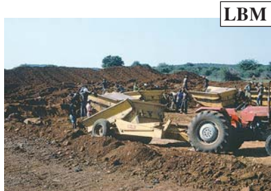
The concept of using labourers and small tractor-drawn buckets is a good example of labour-based methods.
