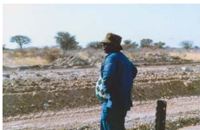
Continuous visual control by skilled staff through the entire operation when processing the base course for LVSRs is essential. Inadequate compaction of natural gravel is often caused by poor mixing, insufficient moisture content or poor final spreading and compaction of the layer.
