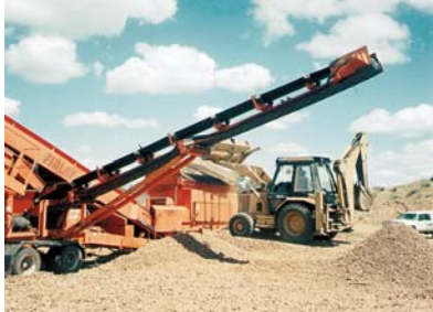
The operational characteristics of the Otta seal are such as to allow the use of as-dug natural gravel which can be screened, if necessary, to remove fines and oversize material.
