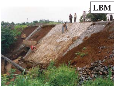
Inadequate culvert capacity, particularly in combination with high embankments can result in severe damage and expensive remedial works.
