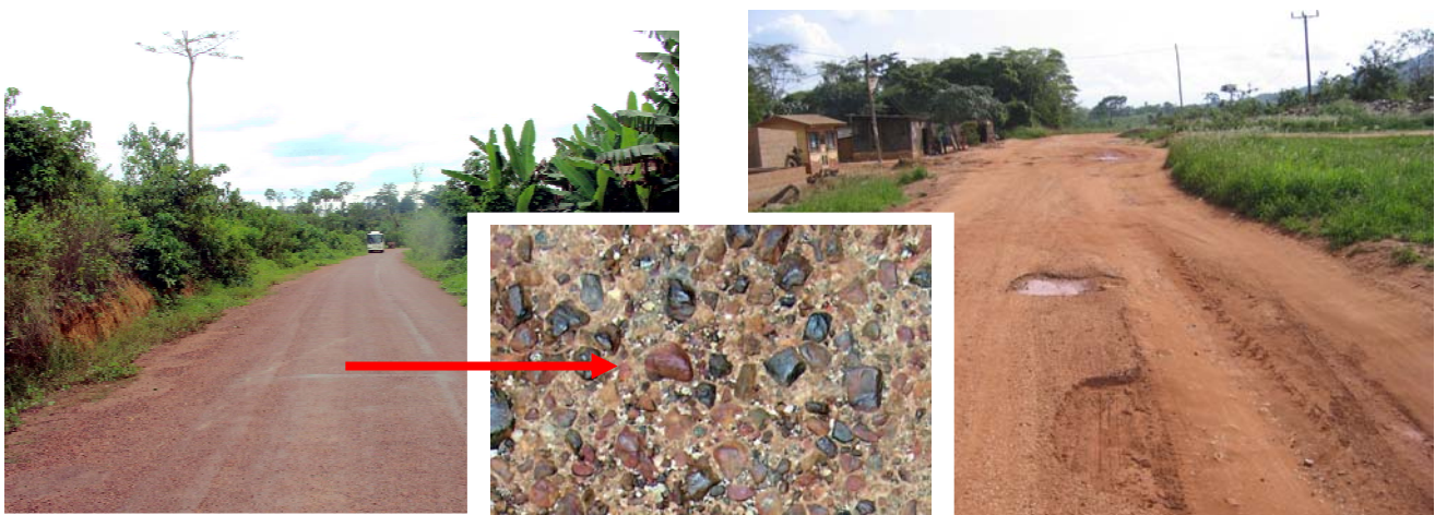
Typical section of feeder road after regravelling and surfacing with an Otta seal
