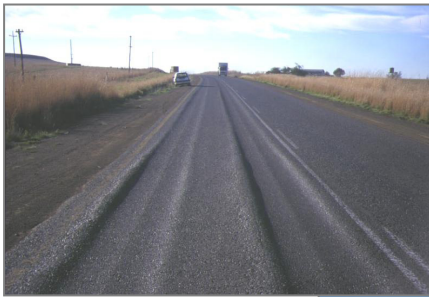
Overloading – The curse of the ESA region's roads
